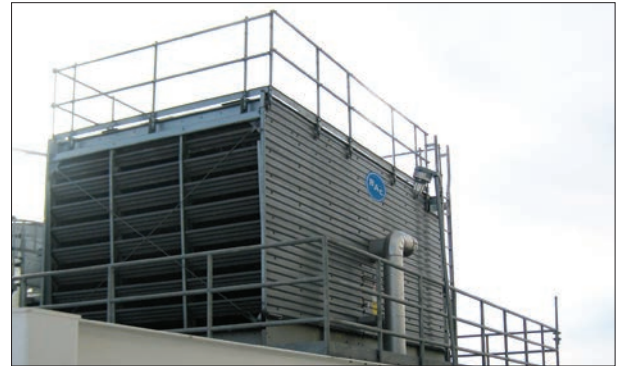
New Series 3000 Cooling Tower
