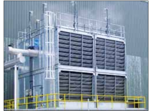
External Ladder, Safety Cage, and Handrail
