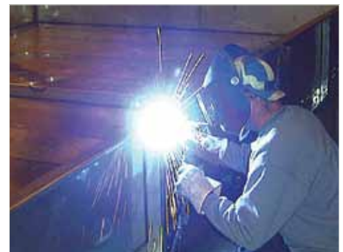
Welded Type 304 Stainless Steel Cold Water Basin
