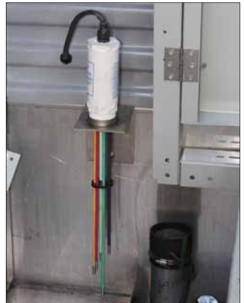
Electric Water Level Control
