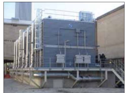
Flexible Piping Arrangement
